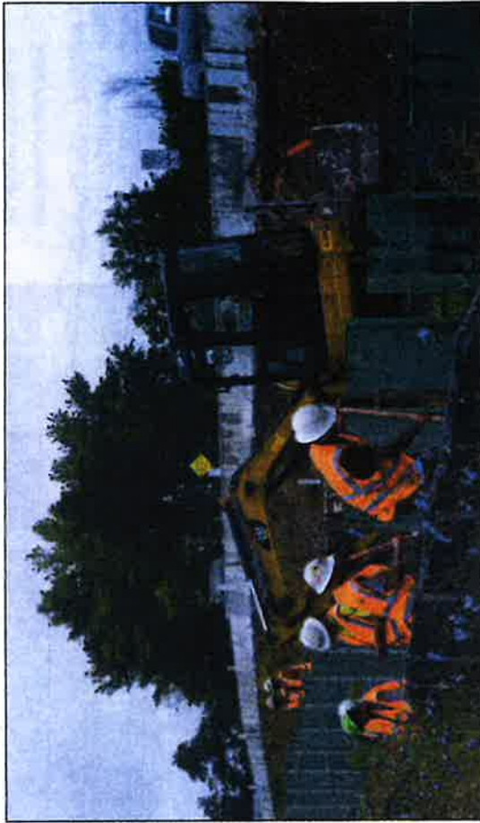
CECIL WHIG PHOTO BY JESSICA MANNETTA The Route 272 bridge over Amtrak lines in North East is one of the Cecil County projects that will receive funding through WILMAPCO.
