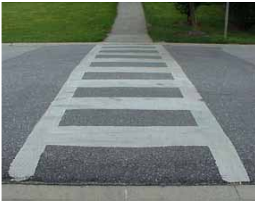
Combined with a raised crosswalk (above), incorporate a curb extension which slows traffic and reduces the amount of time pedestrians are exposed to traffic.
