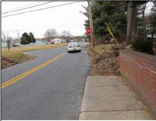
There is approximately 40' of missing sidewalk between the existing sidewalk and High Street.
